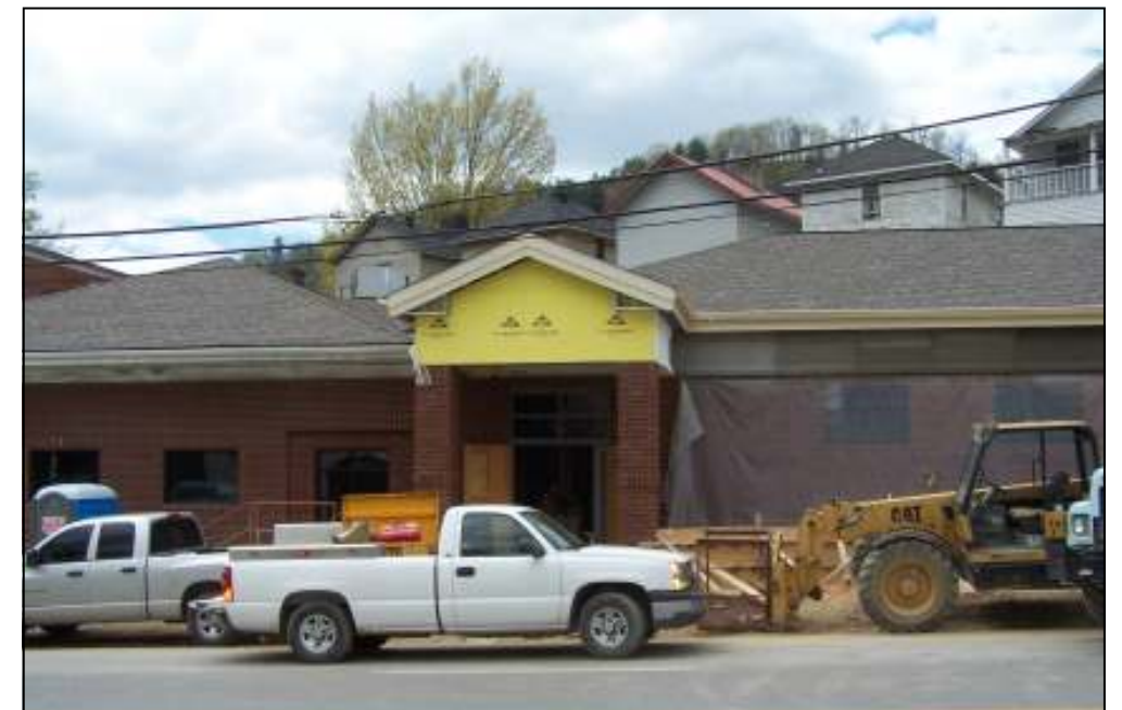
Believe it or not, Starland will be ready for children on June 1. We appreciate the hard work and fast pace of the general contractor, Balis Campbell Inc..
